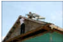
Installing the panels on the roof. The workmen had nothing to protect themselves from the scorching heat or hot tin roof.
